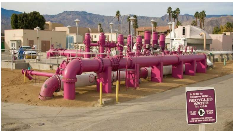
CVWD WRP-10 recycled water serves golf demands in the mid-Valley area.
