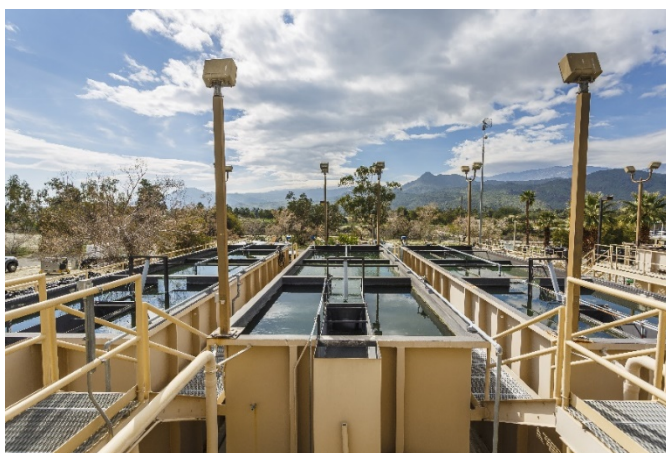
DWA WRP has a tertiary treatment capacity of 10 mgd (11,200 AFY).
