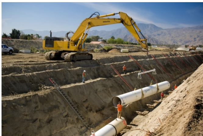
Construction of the Mid-Valley Pipeline in 2009 to deliver Canal water to the Mid-Valley area.
